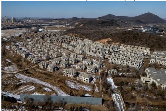
Uncompleted residential buildings at a real estate project on the outskirts of Shenyang in China's Liaoning province earlier this year. Andrea Verdelli/Bloomberg/Getty Images
