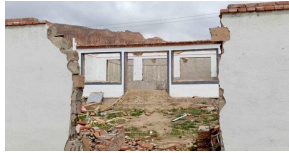
Partial demolition of a structure of Atsok Monastery in Tibet. (Photo: Vera Hue)
