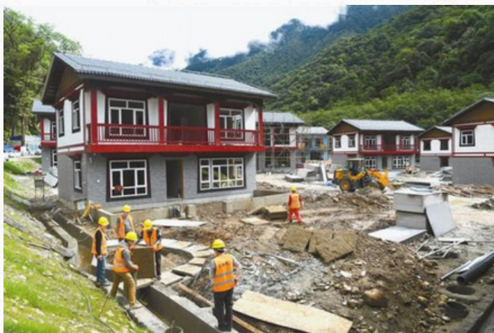
The picture shows the construction site of the resettlement site, Yadong County.
